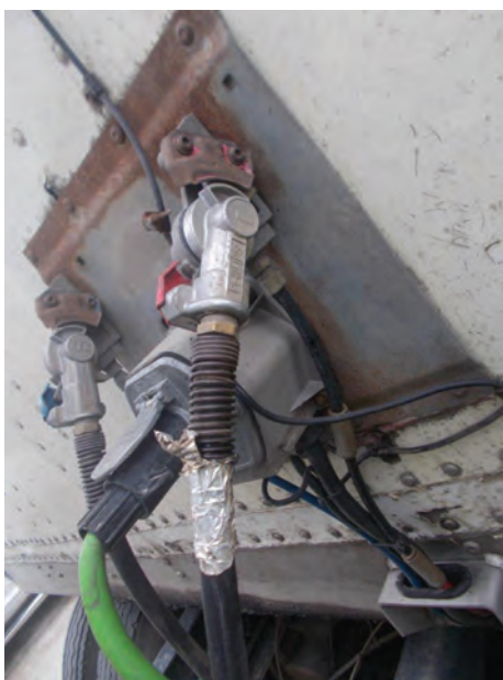
Submitted by Cpl. Williment: The driver put tin foil over a leaking air hose. It was still leaking air during the Level II Inspection. The vehicle was placed out of service.
